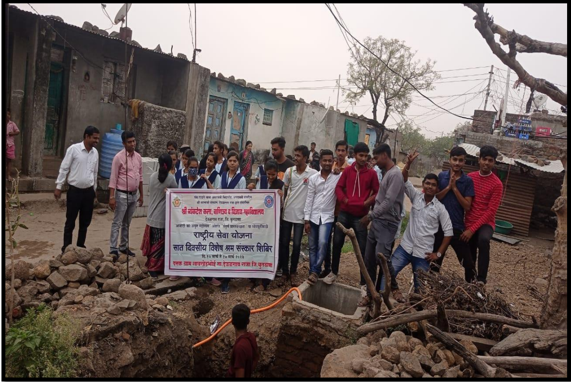
NSS Volunteers digging a Pit for toilet at Saokhed Bhoi during NSS Camp
